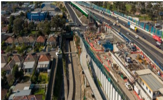
Images: M80 Western Ring Road Interchange and Williamstown Road inbound exit ramp and inbound tunnel area
