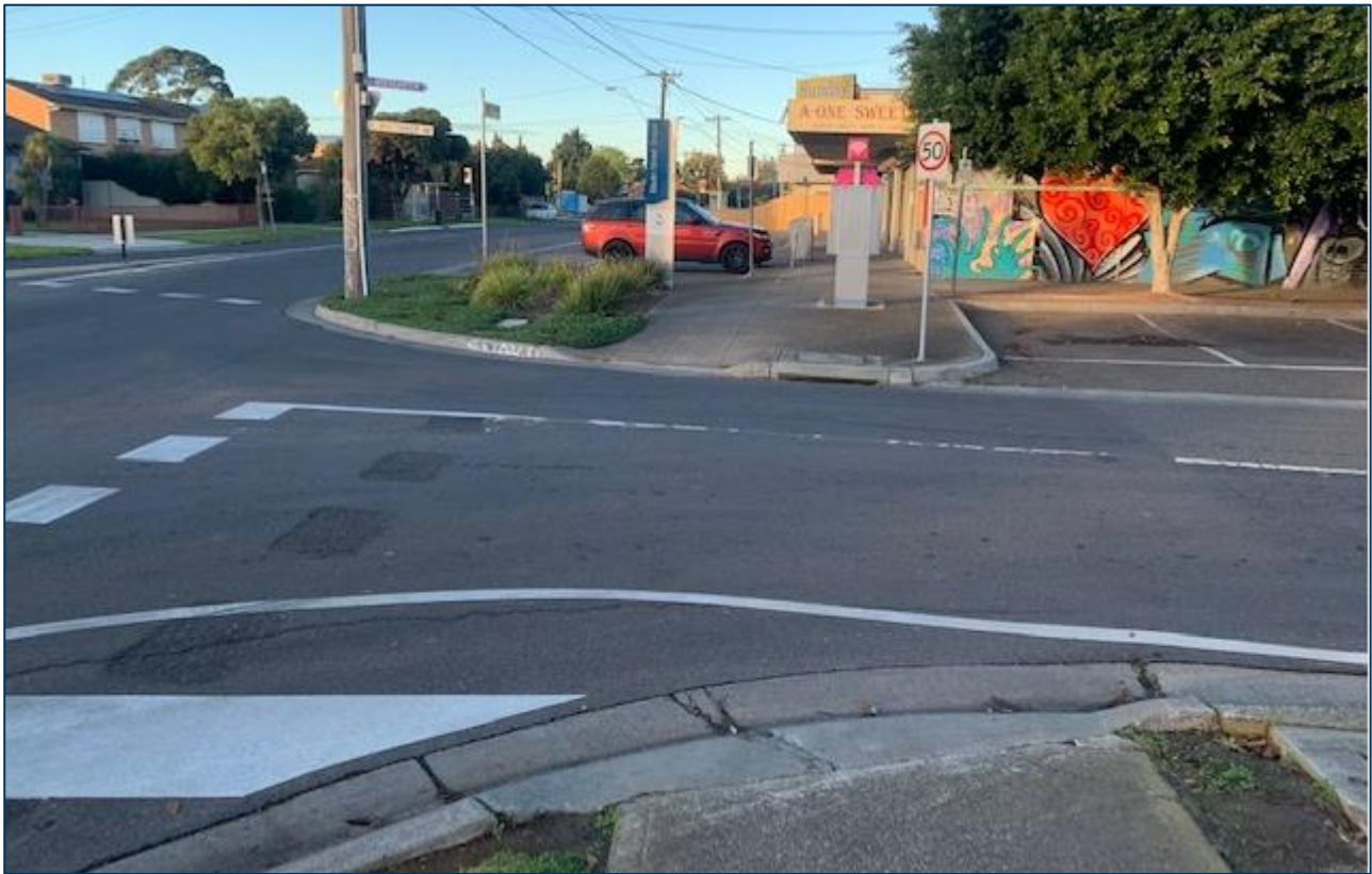
Figure 4-6 Poor footpath connection at the intersection of Bladin Street and Whittaker Avenue
