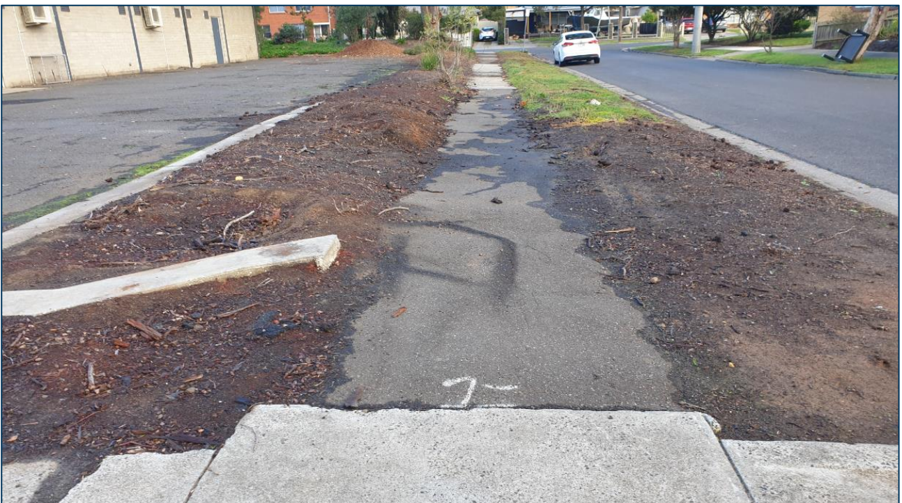
Figure 4-5 Unsafe footpath on Pearce Street
